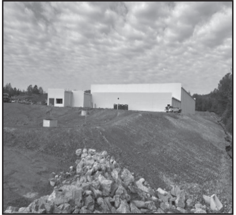
BWXT erected this building in a very short time using large panels of concrete (Courtesy of Ray Smith)
