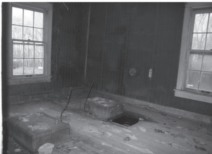
The location where the generator would have set on the two concreted foundations (Photo Submitted)
